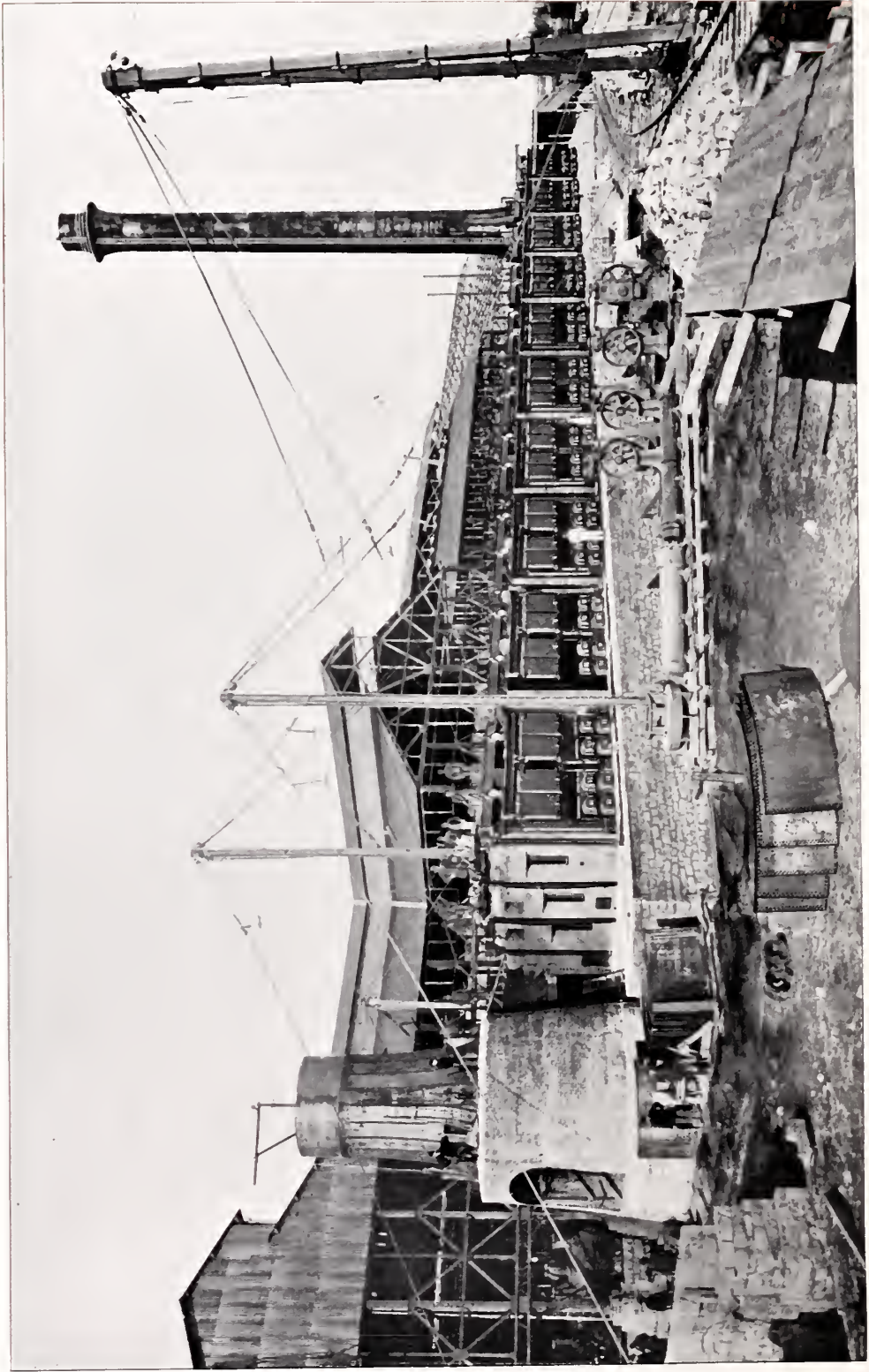
Babcock & Wilcox Boilers at Pennsylvania Steel Co's Works, Sparrows Point, Md. 1st order, 4,000 H. P. in process of erection, 1888. Duplicate ordered 1889.
